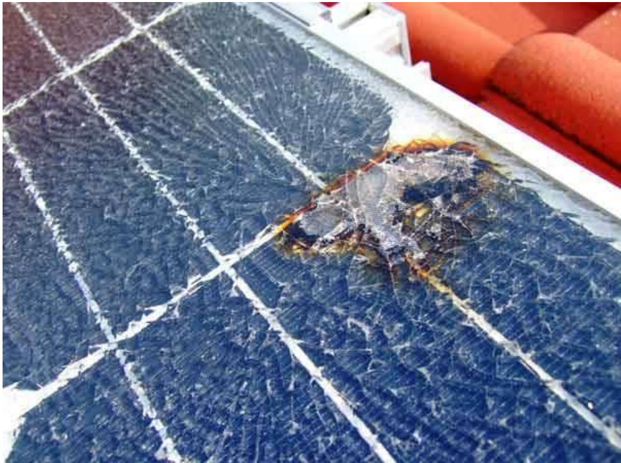
Figure 6: Defected solar panel [5]
