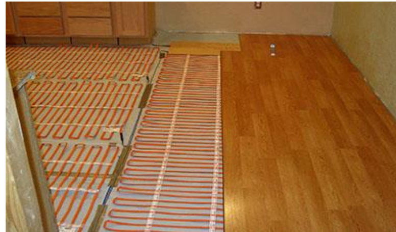
Electric radiant Heating
