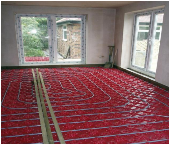
Hydronic Radiant Heating
